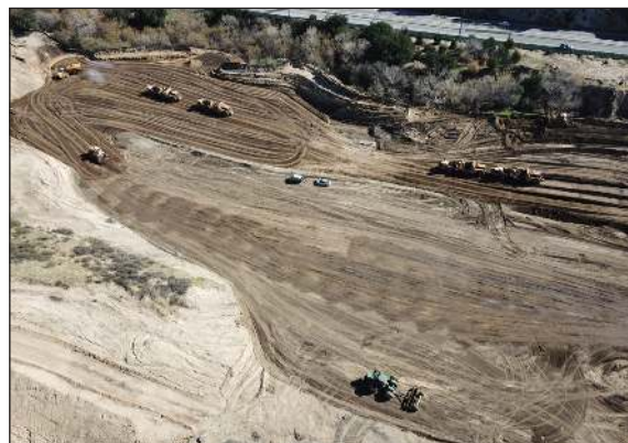
Drone footage shows an aerial overview of the grading project at Needham Ranch in Newhall.
