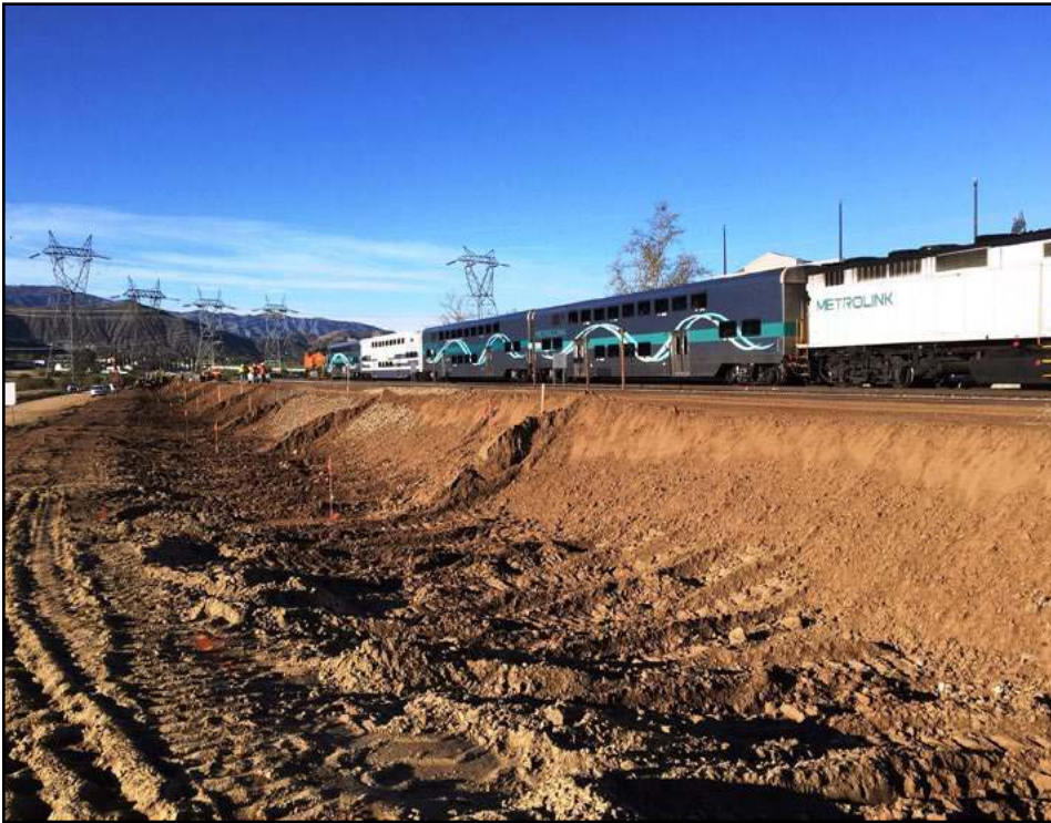
A built-up dirt pad for the new Vincent Grade Acton station platform sits directly across from the existing platform.
