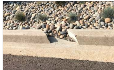
Drainage inlets were created to allow for soil runoff from the bioswale system constructed along Pier J Way.
