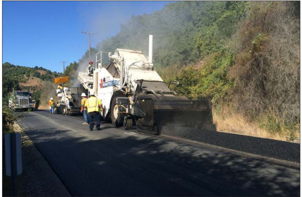
Using bottom dump trucks to place the asphalt ahead of the shuttle buggy helped to speed up and smooth out the process along the two-lane Highway 150.
